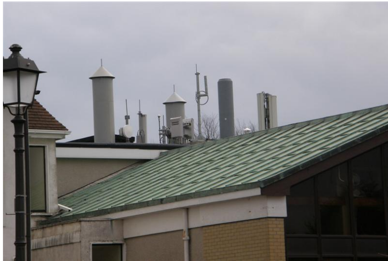
Transmitter Site Photo
